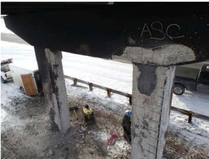
Fire Damaged pier after some heat damaged concrete has been removed
